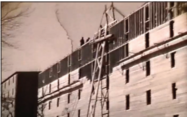
Van Winkle Family Films, ca. 1934–1935, 1947–1952 [Mss. A V285] These digitized family films document the Van Winkles of Louisville, who were best known for their leadership in the Stitzel-Weller Distillery in Shively. The films depict the ca. 1934–1935 construction and grounds of the distillery, the home of the Van Winkles, and family leisure activities. (Donated by Sarah Van Winkle Campbell)
